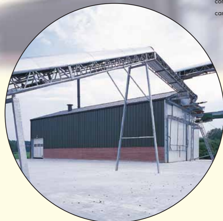
Overview of composting tunnel
