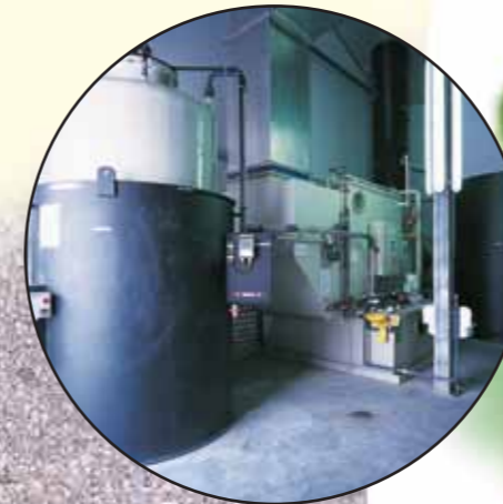
air washing system and spraying tank
