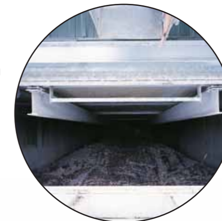
Loaded manure tunnel
